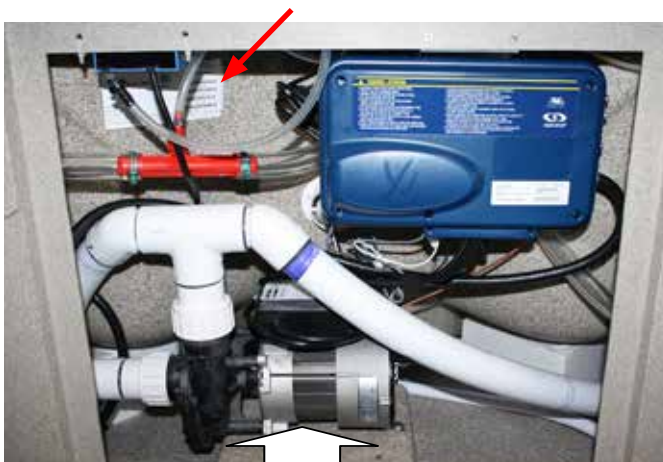
110 Volt Equipment Compartment
